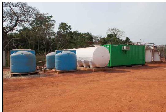
STATION D'EPURATION DE LA BASE A BOUE ACTIVEES
